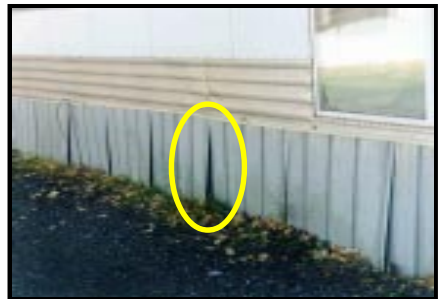
Fix gaps in trailer skirtings
